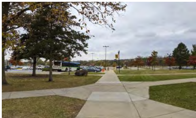
Patched Concrete on West Side of Main Building
