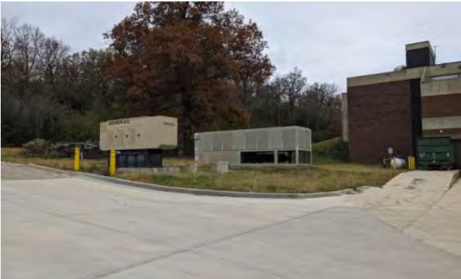
Generator and HVAC Equipment
