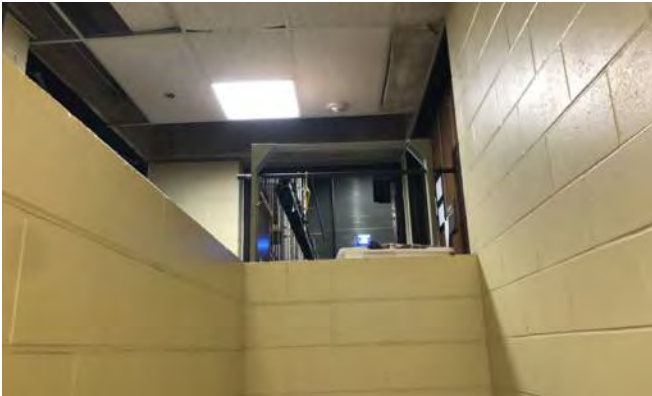
Damaged acoustical ceiling
