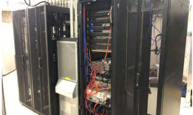
Server Room Accessed from H1317
