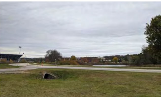
Culvert Connections for Stormwater Conveyance
